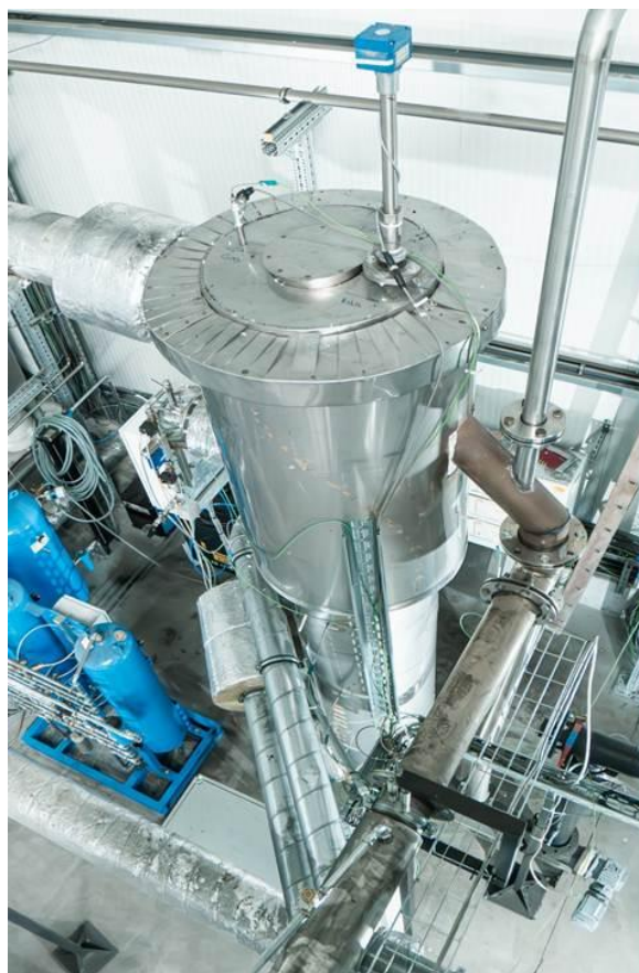
Figure 1. Pilot unit at Fraunhofer UMSICHT industrial facilities..
